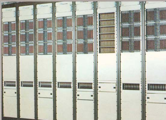
900 SERIES ROUTING SWITCHER AT PACIFIC BELL
